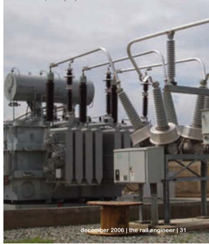
A pair of Infeed 115kV/13.8kV 24MVA transformers, HVCB(SF6).
